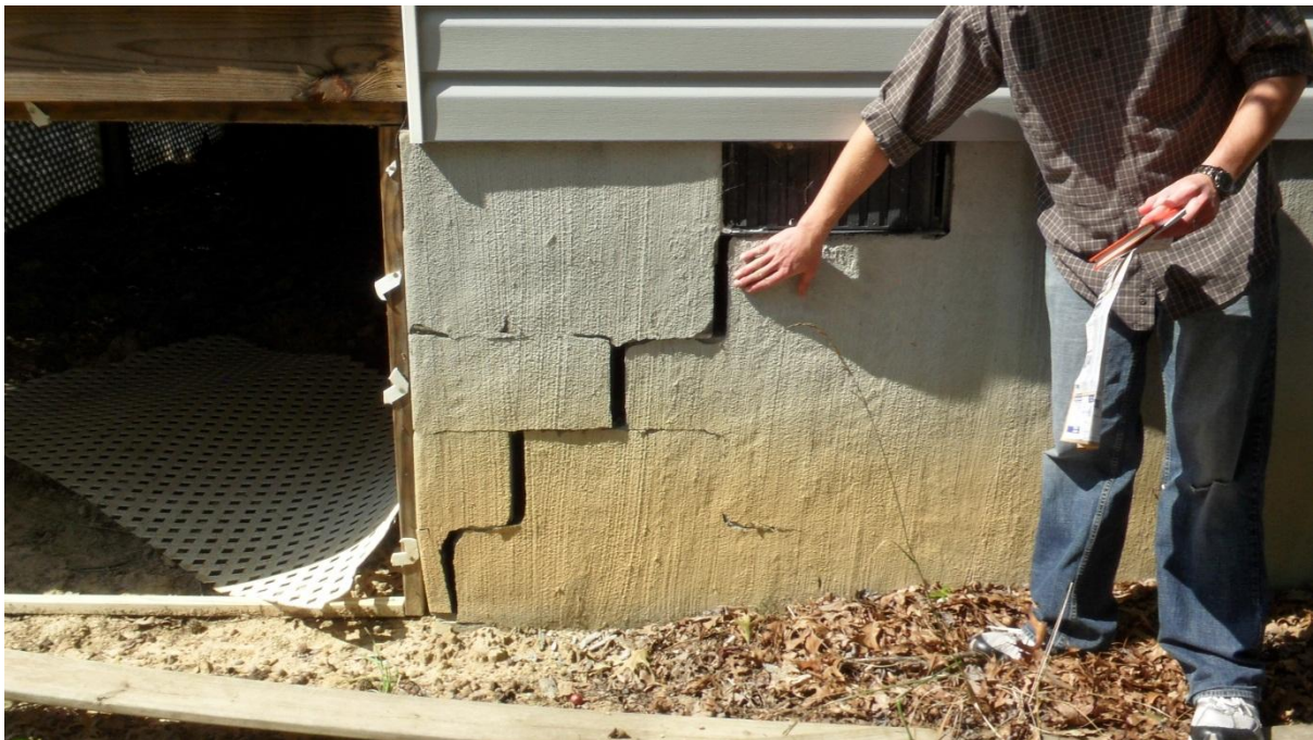
Figure 51. Typical damage to block foundation walls (37.9790, -77.9692).
