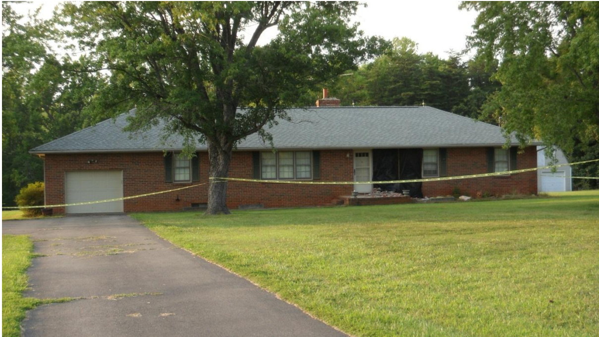
Figure 56. Representative severe damage to brick façade (37.8878, -78.0267).
